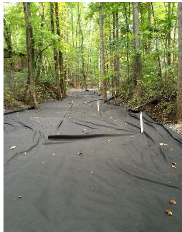
One section of the springs mid-construction of the treatment system. White pipes go down to connect to air sparging pipes.
