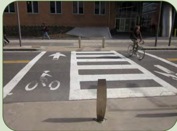
High volume multi-use crosswalks, such as one connecting to a school or park, may require separation of uses to avoid user conflict.
