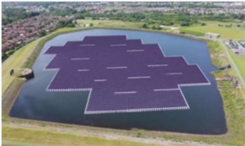
FPV on drinking water reservoir, Manchester, England.
