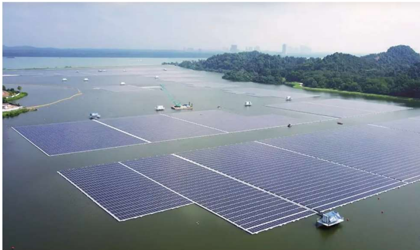
Tengeh drinking water Reservoir, Singapore 60 MW floating Solar
