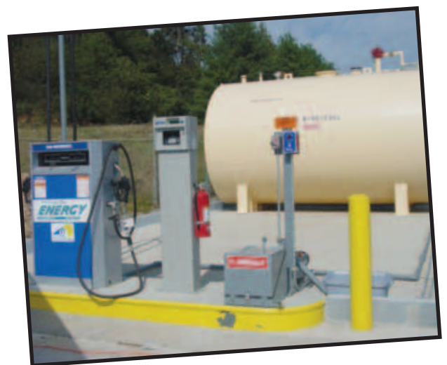
Buncombe County's bio-diesel pumping area is located at the Transfer Station.
