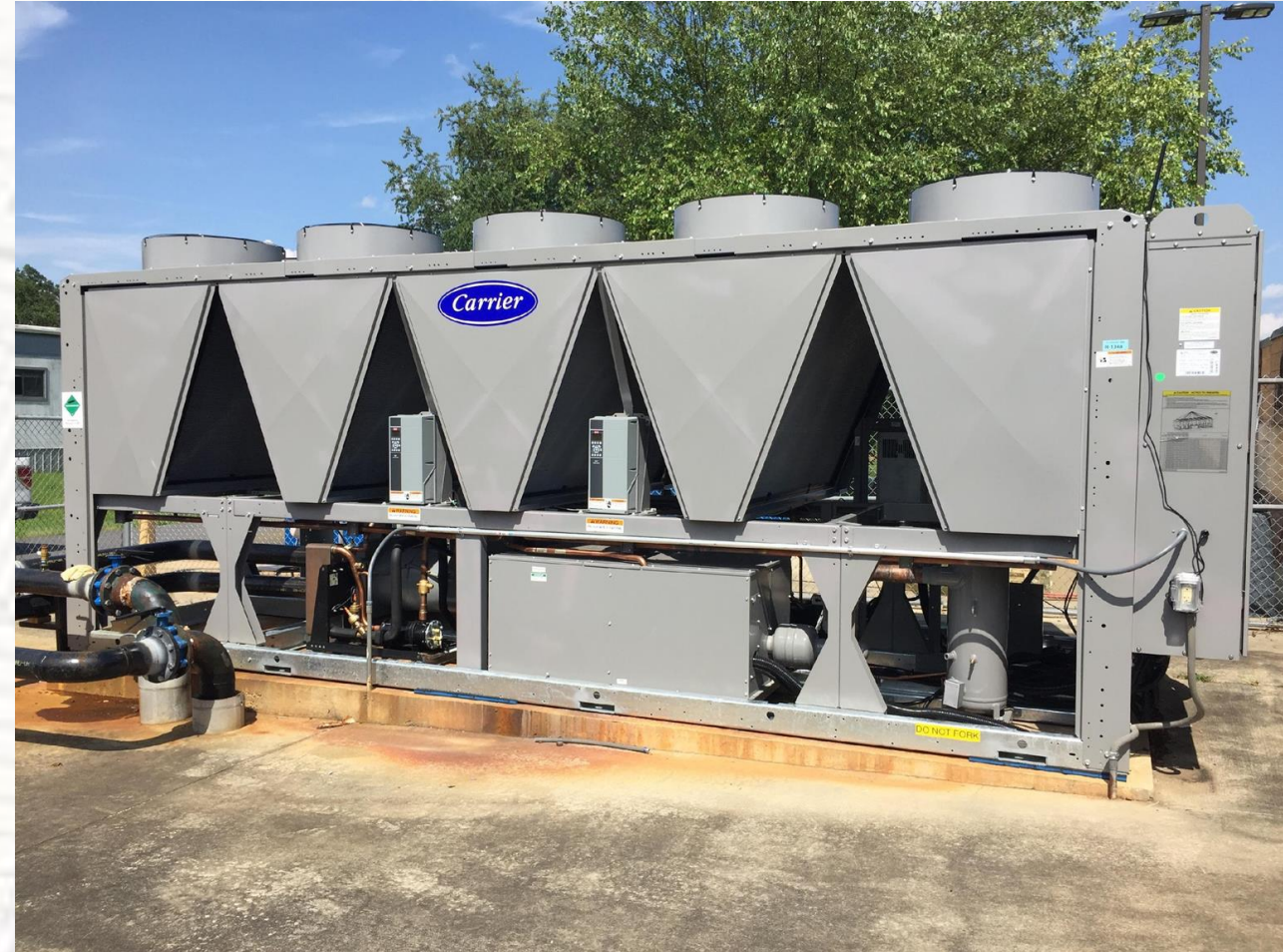
Carrier air-cooled 30XV High-Efficiency Chiller, Avery's Creek
