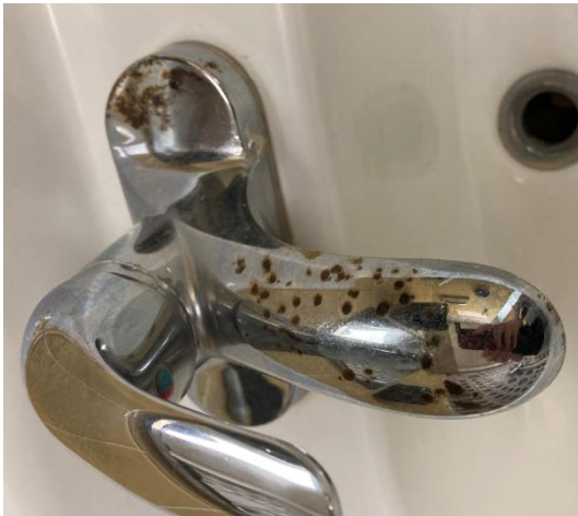
Faucet rusted in ELC bathroom.
