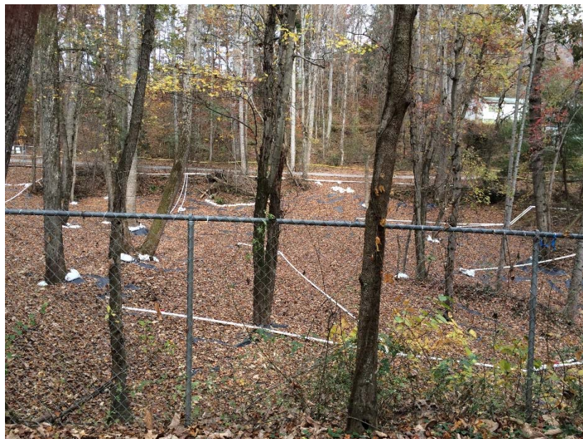
Photo of treatment system piping in springs in November 2014
