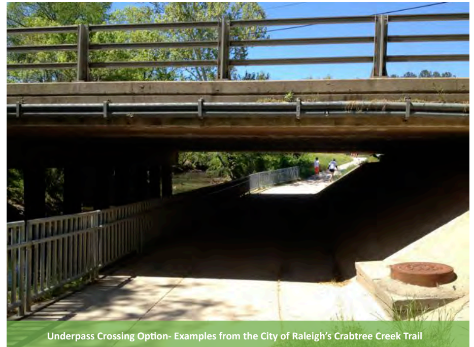
Underpass Crossing Option- Examples from the City of Raleigh's Crabtree Creek Trail
