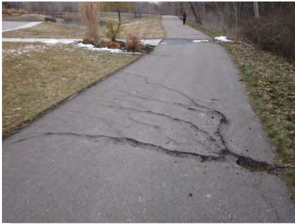
The combination of a wet climate, winter freeze/thaw cycles, and tree roots can create significant damage to greenways, causing potential safety hazards for all users.
