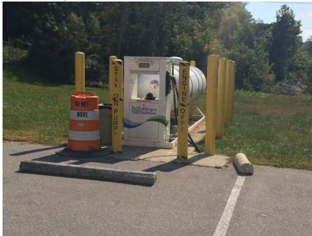
Figure 15: LPG Fueling Station
